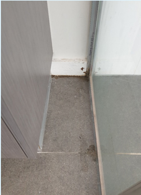
Damaged timber skirting and vanity kickboard in bathroom.
