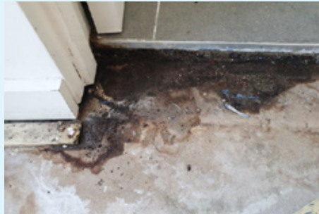
Carpet pulled back at the doorway to uncover extensive dampness and mould growth.
