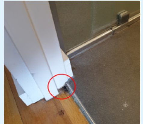
Picture shows rotting timber floor. Water was found to be coming from the shower that had no shower perimeter water stop and an incorrectly installed perimeter water stop.
