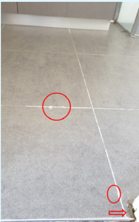
Damaged timber doorjamb to the right and leaching through grout joints.
