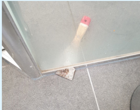
Sliding the scraper under the screen with little to no resistance is an indication of no water stop 5 mm above FFH.
