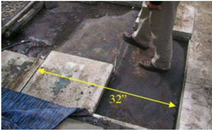
Figure 3: Large "water-bed" type blister lifting pavers.
