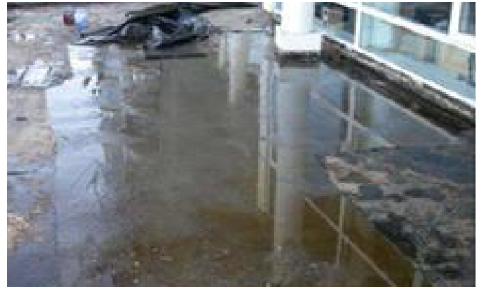
Figure 4: Water beneath blistered membrane over entire deck.
