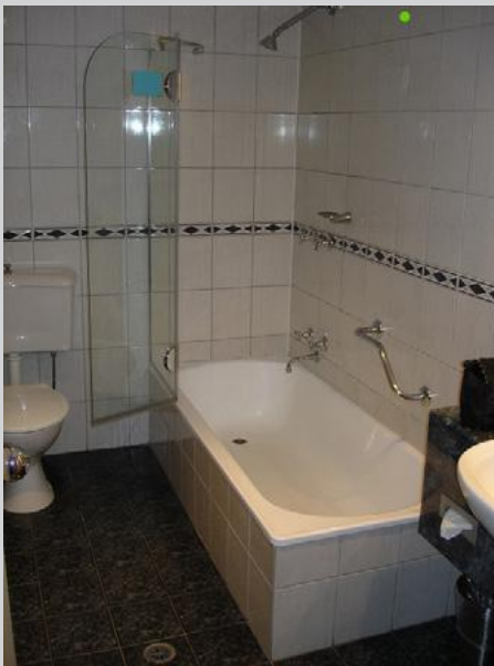
Figure 1 - Shower installation over a bath in this installation the shower screen is hinged so that when it is closed it will extend more than 900 mm from where the shower rose is fixed into the wall. If the distance is less than 900 mm then splash water will not be confined to the bath and the waterproofing will need to be extended onto the general floor area of the bathroom and be drained to a floor waste as shown in figure 2.
